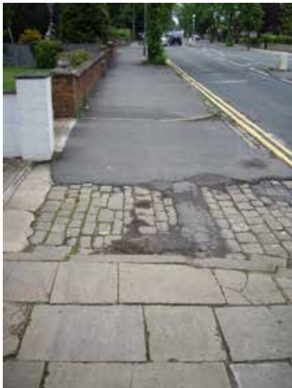
Fig. 3.24 Stone paving lost to tarmac and setts covered
