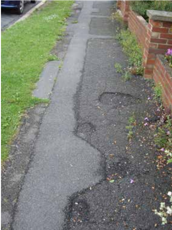
Fig. 5.7 Irregular footpath due to degradation
